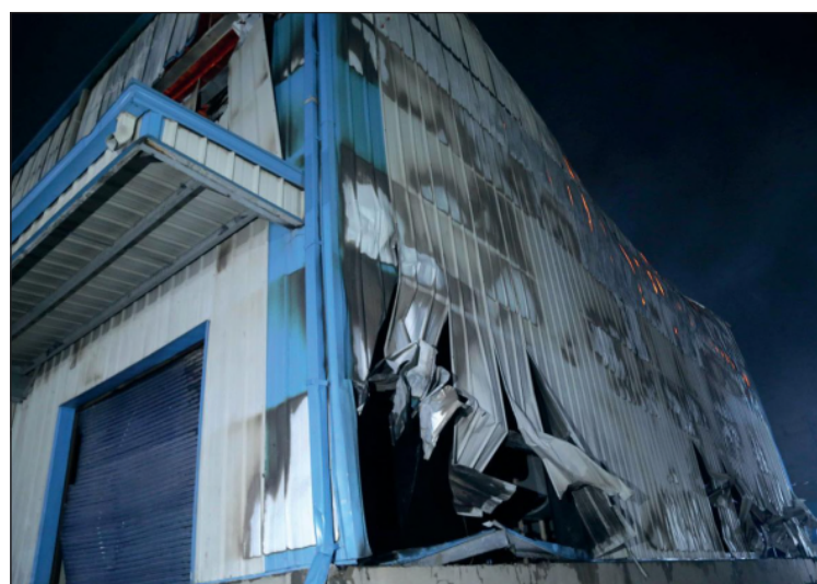
Damage is seen after a fire broke out at Nandan Denim, one of the largest denim suppliers in the world, in Ahmedabad, India on Feb. 8, 2020.
