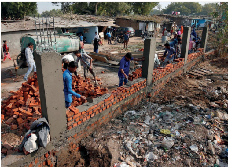
Construction workers build a wall along a slum area as part of a beautification drive along a route that U.S. President Donald Trump and India's Prime Minister Narendra Modi will be taking during Trump's visit later this month, in Ahmedabad, India on February 13, 2020.
