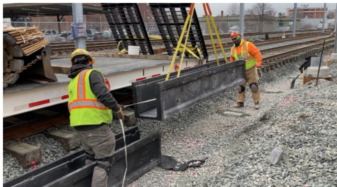
Chapman crew installing cable trough along the tracks at Green Line Extension (GLX) Project
