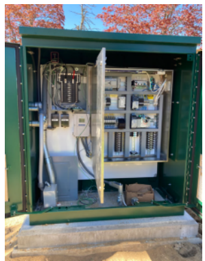
Harwich Pump Station Control Panel recently installed
