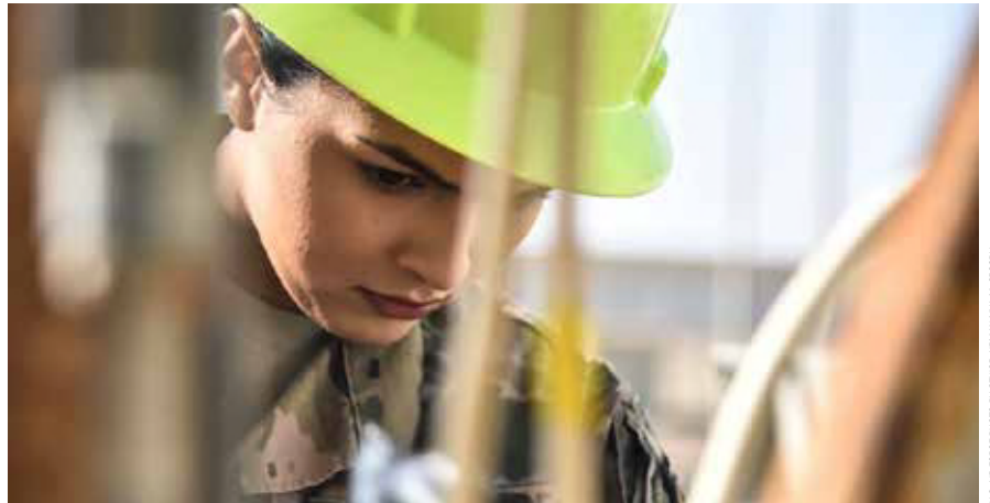
Senior Airman Angelica Gutierrez, 380th Expeditionary Civil Engineer Squadron electrical systems journeyman, identifies wires in a junction box at Al Dhafra Air Base, United Arab Emirates.
