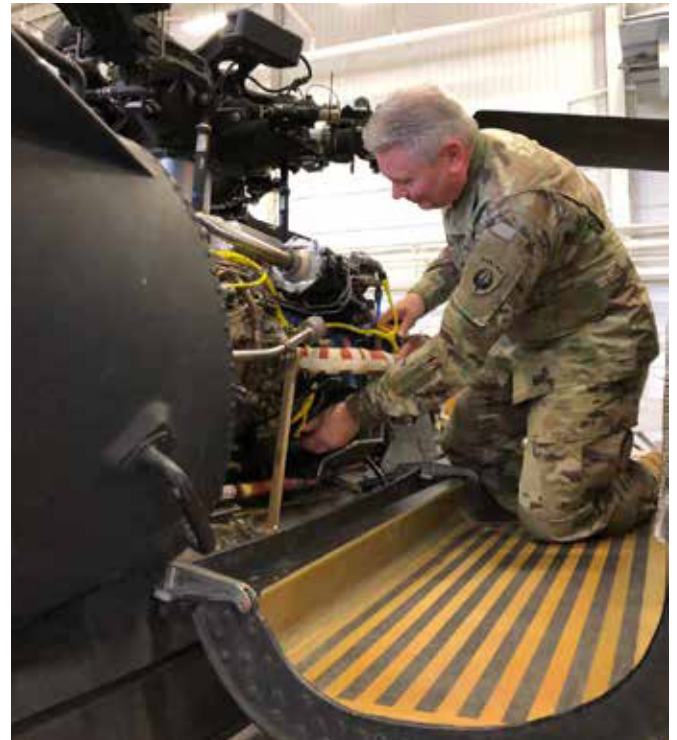
CW5 Robin Vozar, the longest serving Night Stalker, inspects a repair at the limited Depot facility at Fort Campbell on an MH-60M.
