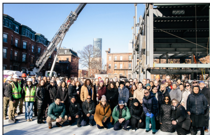
Attendees of the beam signing and raising pose in front of La CASA’s future site.
