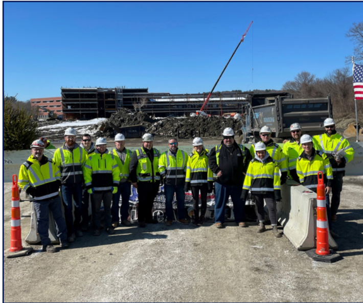
Members of the Skanska USA Building team gathered on Friday, March 4, 2022, to celebrate the topping out at Belmont Middle School.
