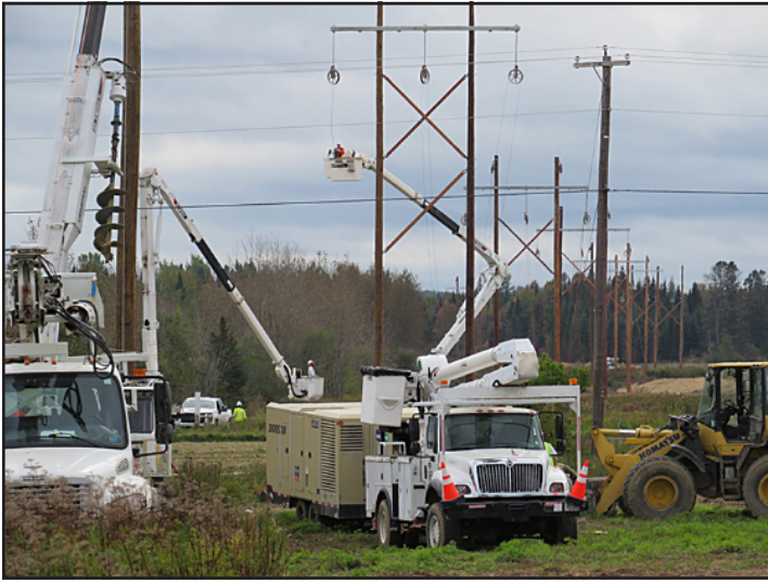
Homeland Power & Utility's crew of IBEW Local 104 linemen modernized more than 5 miles in the Transmission Line 1176 modernization project in Presque Isle, Maine for Versant Power, setting 49 new double and triple pole structures.
