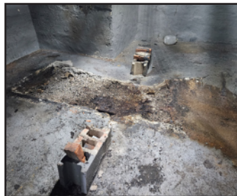
Floor under leaking tank.
