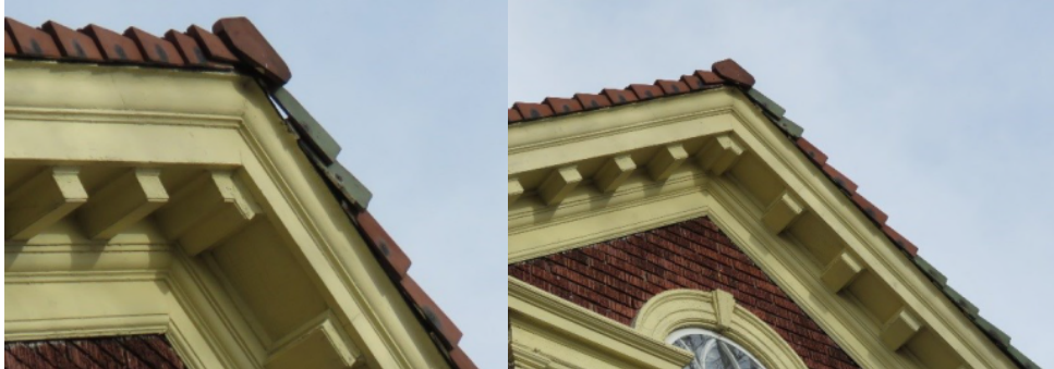
Notice unmatched gable rake tiles located at gable end.
