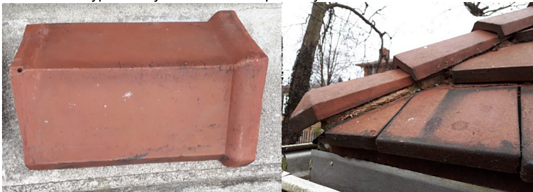
Plan view of Ridge Tile Cap (end), and close up of roof hip tiles (without lip)
