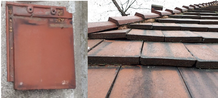
Plan view of typical clay tile and close up of clay tile on roof
