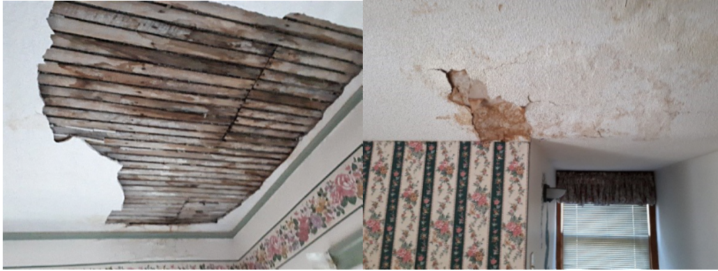
Interior damage to ceiling due to roof leaks
