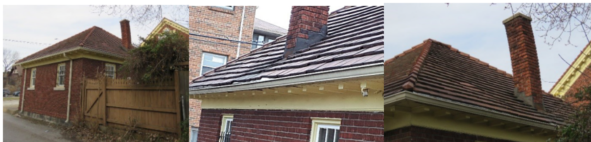
Slipping tiles and tilting chimney at rear of garage roof
