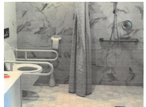
CLEAN DESIGN: Universal design bathrooms feature curbless shower stalls and shower seats for the chairbound.
